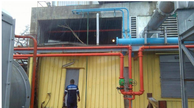
Pernix's Vuda Power Station suffered damage during the storm. Shown above, a portion of the wall louvres collapsed from the heavy wind, letting rain into the building.
